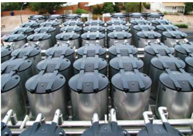
CALMAC Ice Storage tanks located at CRB Plant
