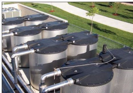
Eight large insulated tanks store ice made during off-peak hours when electrical rates are lower.
